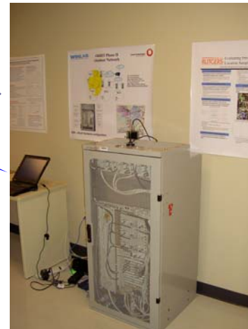
Lucent IP Base Station Router at WINLAB
