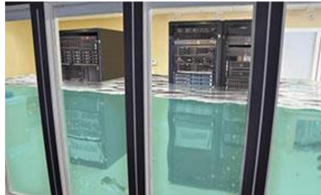
Flooded datacenter due to burst water pipe - NYU
