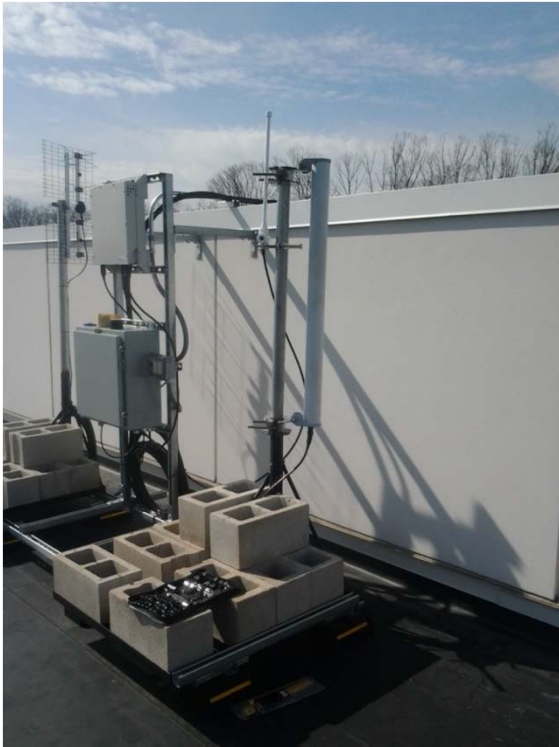
Roof mounted Antenna
